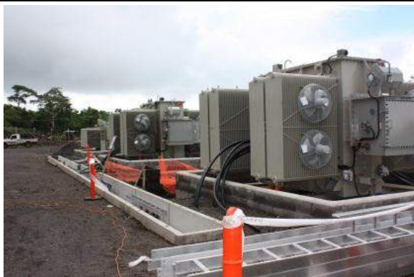
Above : Transformers outside the Fiaga Power Station shortly after installation.
