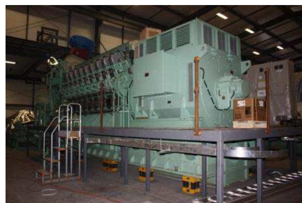
Above: One of the generators installed at the Fiaga Diesel power station.
