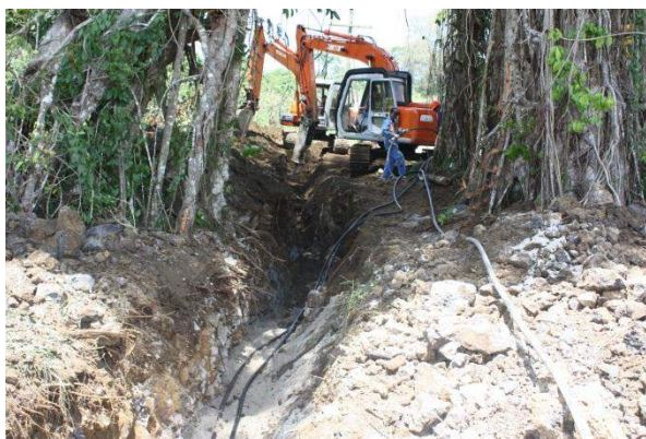
Above: Laying of conduit for underground 33kV lines connecting electricity supply at Fiaga.
