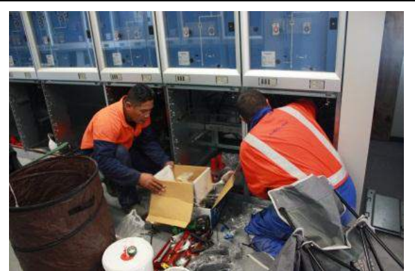
Above : Contractors North Power staff with EPC staff during the installation of switchgear panels at the Fiaga Power Station.
